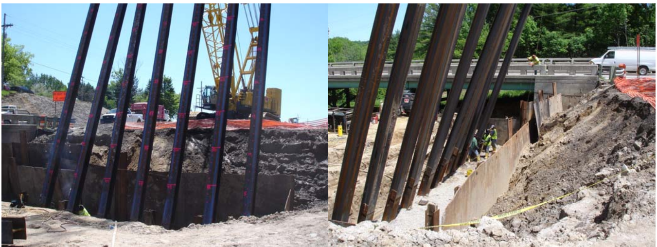
Marks on the pile to show how deep they have been driven
